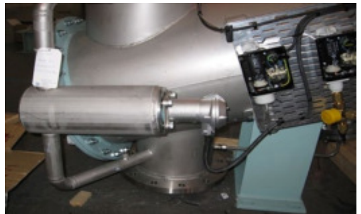
Customized stainless steel float chamber with Trimod'Besta level switch for low level alarm.
